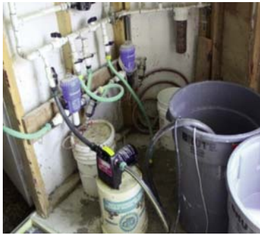
Fig.81.20: Submersible pumps can be used to inject proper concentrations of line cleaners into water systems.
