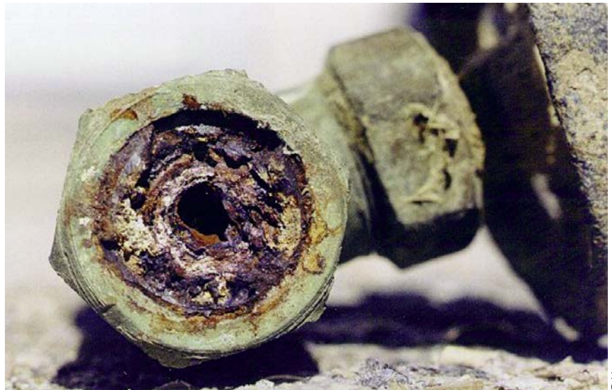
Fig.81.34: Fouling of water lines alters the flow of water.
