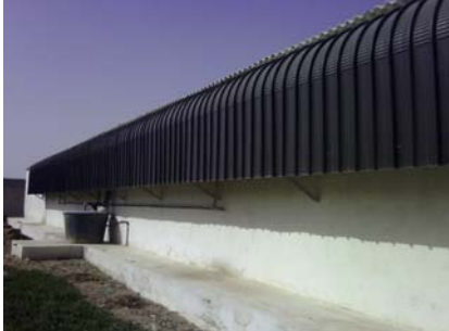
Fig.7.17 & 7.18: Cooling pad. Exterior appearance with partial recovery of water and interior view.
